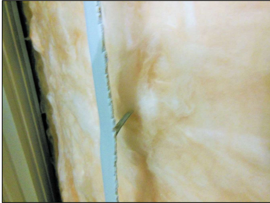
Foam on Insulation Support and Banding
