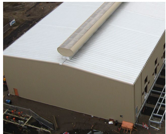
Example of metal roof and wall panels on a building under construction.
